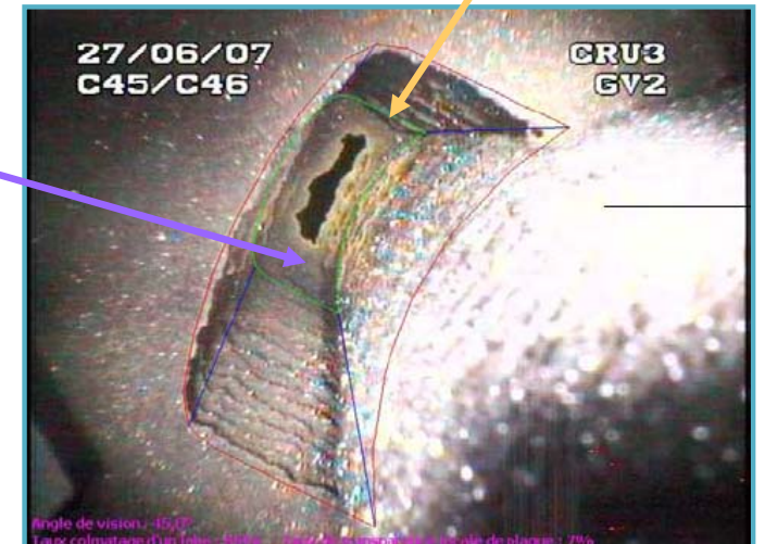
Clogged quadrefoil shaped hole
