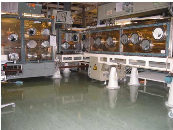
Fig.3 Typical glove boxes intallation at the Belgonucleaire MOX plant [2].
