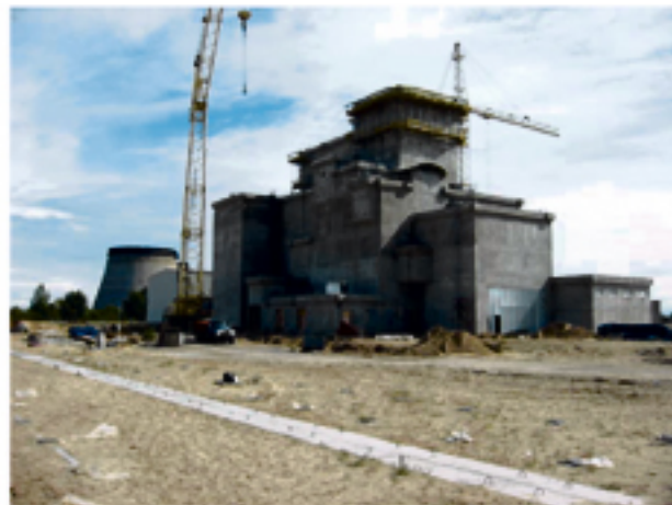
Progress of construction work of the Chernobyl Spent Fuel Interim Storage (ISF-2) in September 2003
