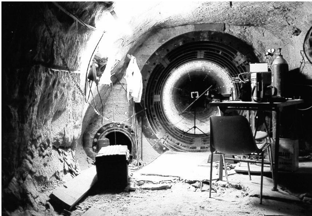
Figure 2: View into the bulkhead drift showing the permeability measurement system (on the right)
